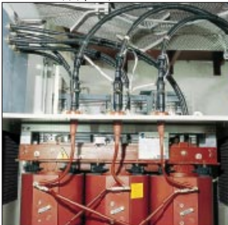
HV and LV connections from above.
