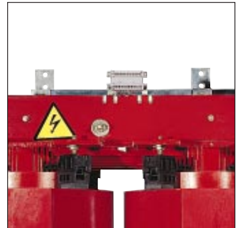
terminal block connecting the T digital thermometer to the PT 100 sensors
