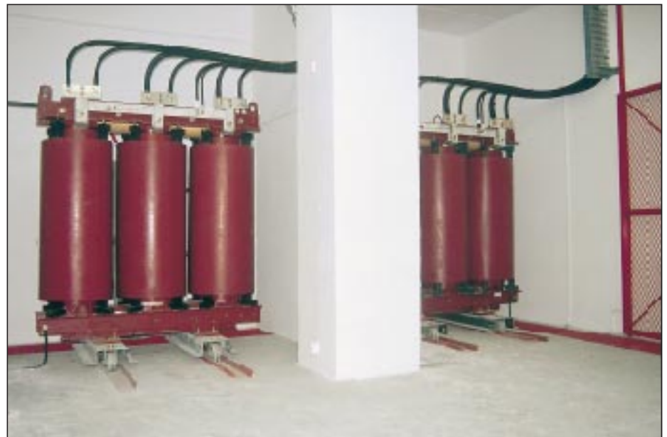
Standard HV and LV connections from above
