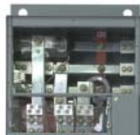
Figure 25: Top-Located Main Lug Compartment
