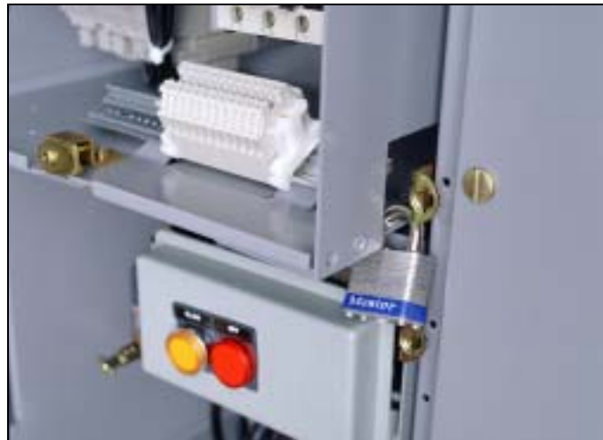
Figure 33: Locked Out Device
