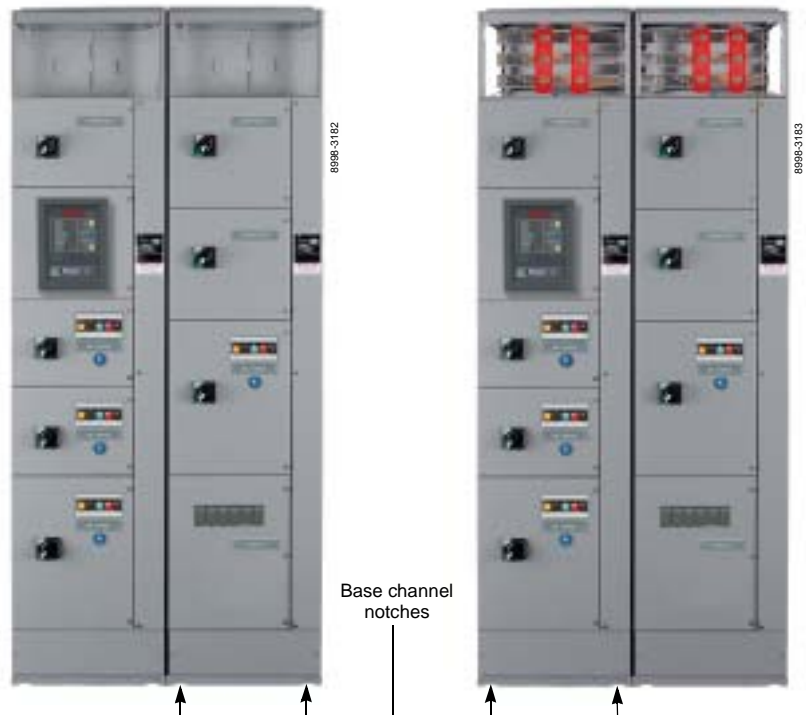
Figure 5: Horizontal Wireway Covers Removed (left) and Two-piece Bus Barriers Removed (right)
